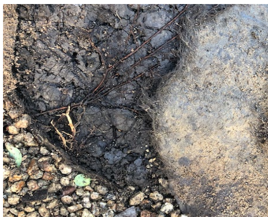
Roots found attached to fabric
